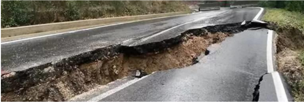
Effects of a deep-seated landslide
